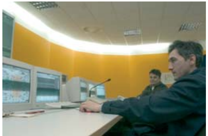
A new computerized control room at Nikola Tesla A power plant
