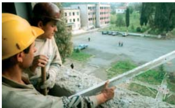
Renovation work being carried out at the Police Academy Arben Zylyftari, Tirana
