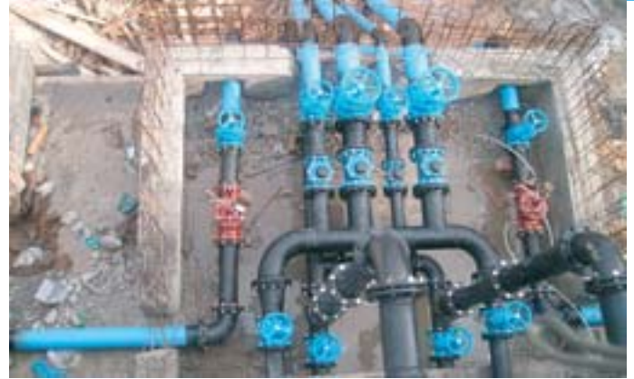
Renovated water transmission system has helped boost local water supply by 30 per cent
