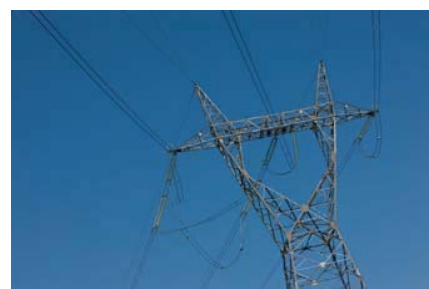
Existing 400 kV lines in the former Yugoslav Republic of Macedonia
