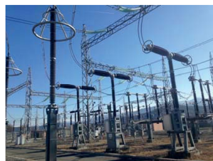
Modern substation in Elbasan, Albania.
