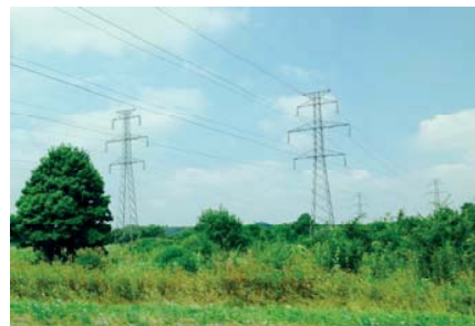
Low voltage transmission lines on the Kragujevac – Kraljevo route
