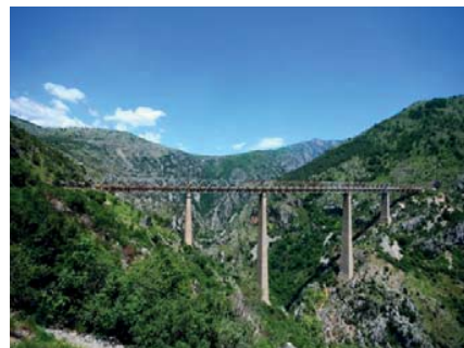
View of the longest bridge on the Podgorica – Bar railway line, on Mala Rijeka.
