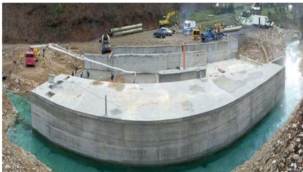
Small Hydro Power Plant in Bistrica, Montenegro
